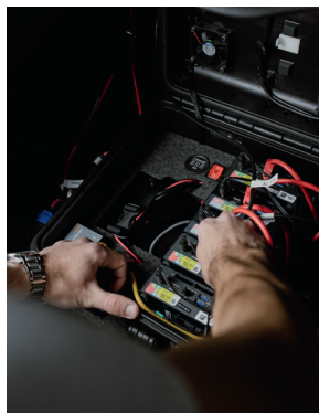
A special control system monitors the smartphones and logs the measurement values they collect.
