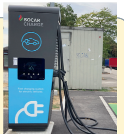
Focused: The charging stations do their job without complaint.
