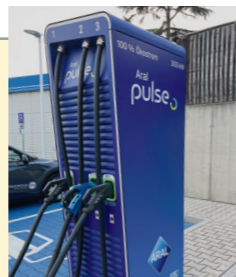
Electricity pumps: Overall, charging at Aral went well.
