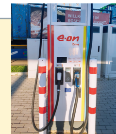
Charging blockage: One station simply did not want to charge.
